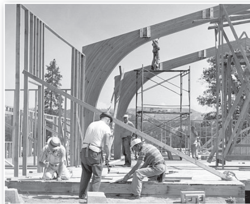
Fresno Flats Historic Village and Park Research Library/Special to Sierra Star Construction of the Oakhurst Community Center in 1964.
